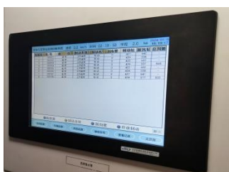
列车监控显示屏 Train Monitoring Display Screen
